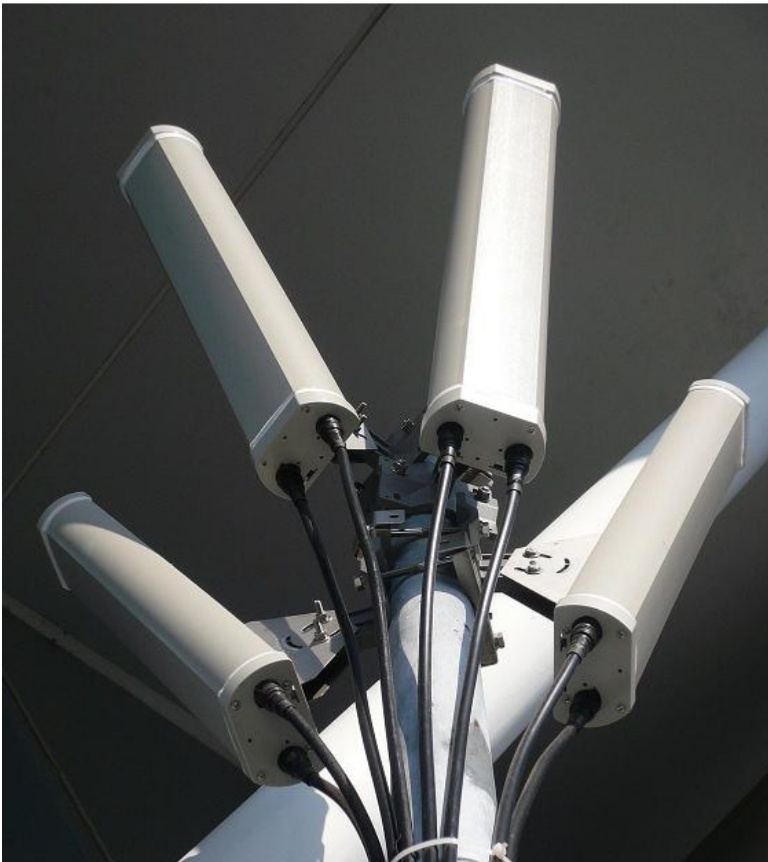
Figure19. RF cable connection from panel antenna
