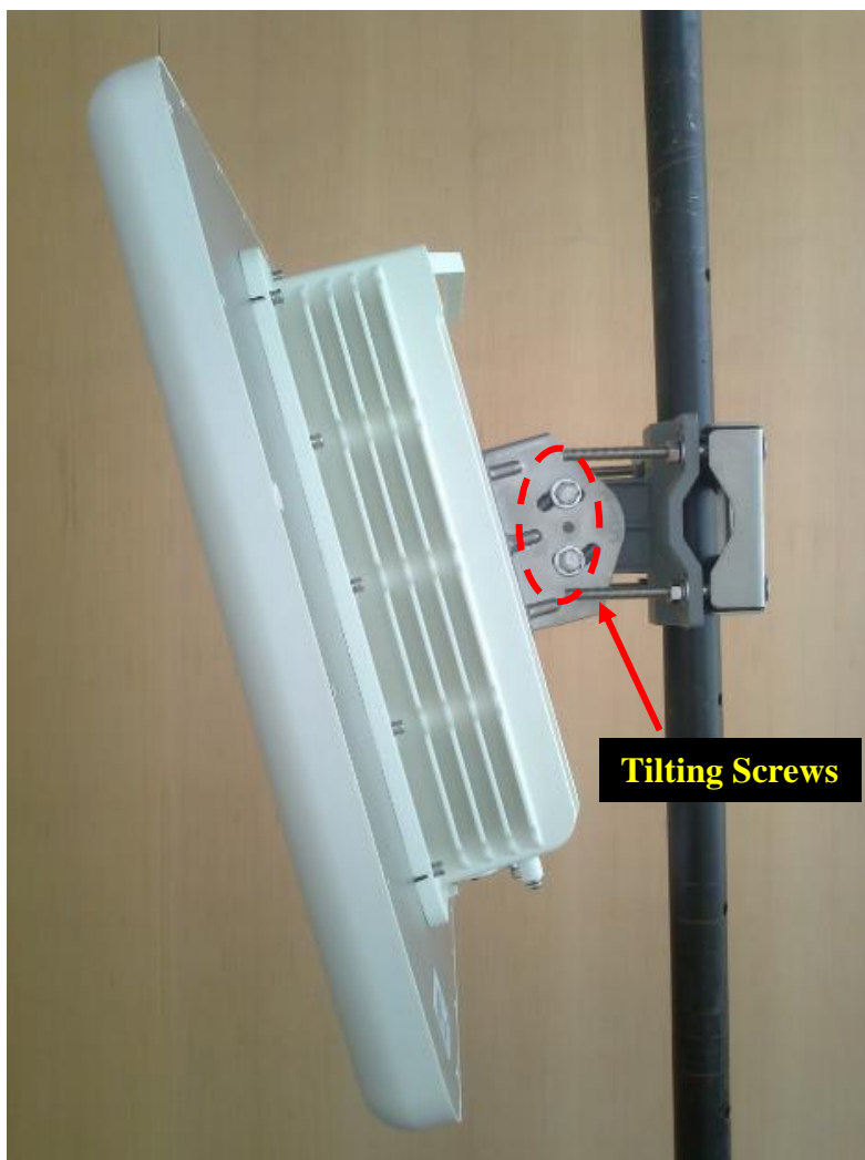
Figure 9. Antenna Mounted on Pole
