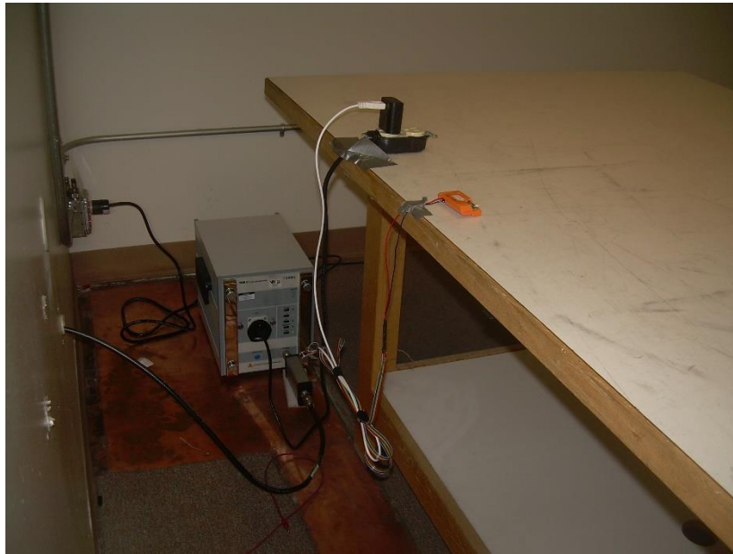
Photograph 8: Back View Conducted Emissions Worst Case Configuration
