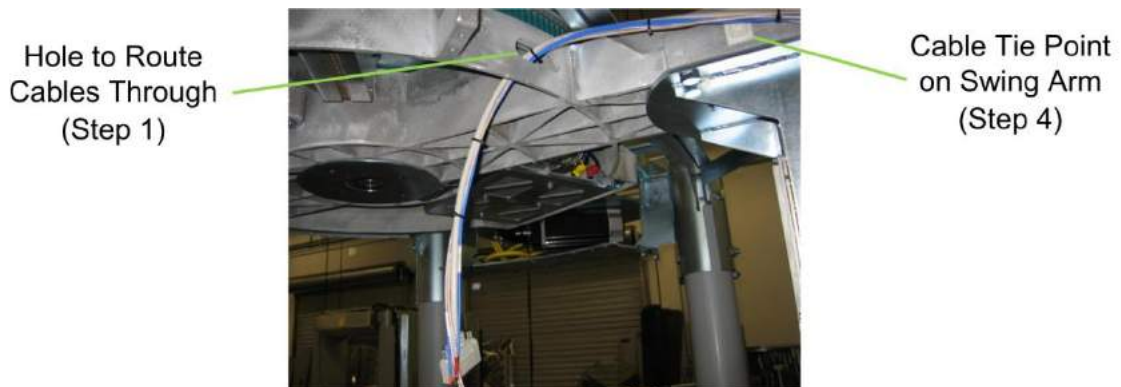
Figure 55: Cables Routed Through Swing Arm Hole
