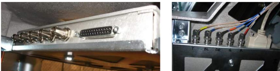
Figure 57: Connectors on ISU and Cables from Mast Connected to ISU
