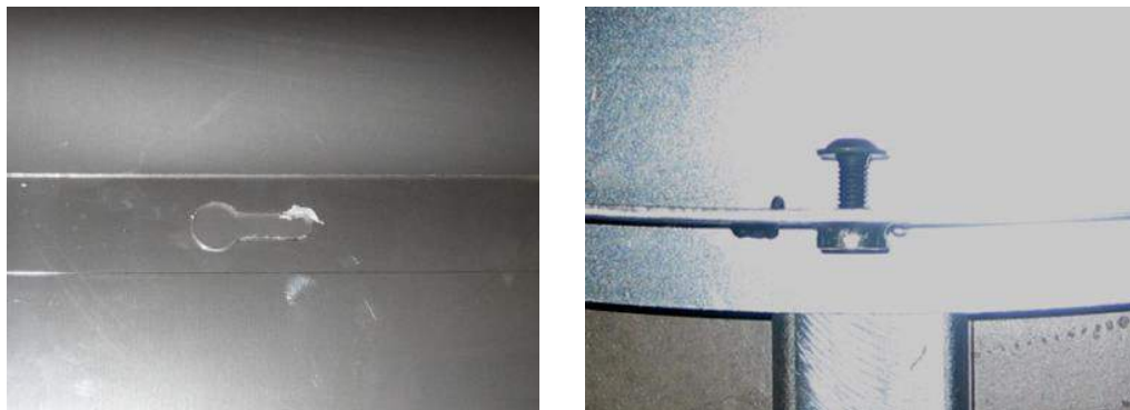
Figure 86: Inner Radome Slotted Hole and Screw Sticking Out
