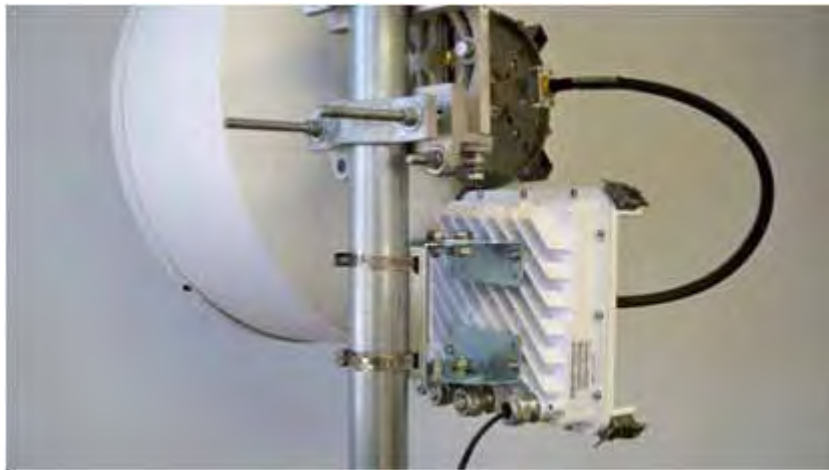
Figure 12 Remote-mount pole mounting mechanics, vertical orientation
