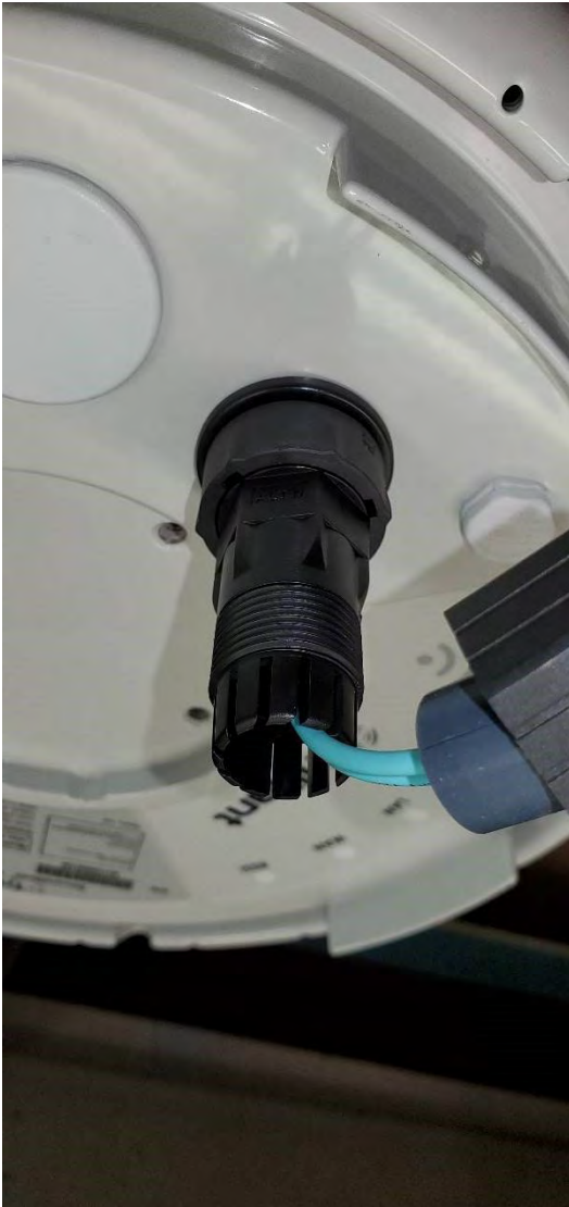
Figure 28: Fiber Optic cable with bayonet nuts attached and secured.
