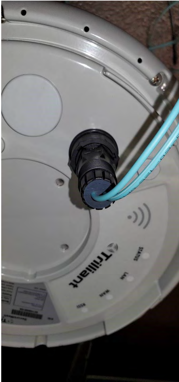
Figure 29: Fiber Optic cable with sealing grommets in place.
