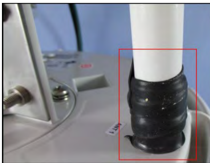
Figure 39: Inner layer of electrical tape on antenna connection
