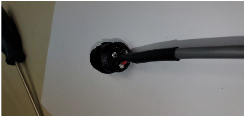
Figure 21: Fiber Optic cable soldered to the DC Connector.
