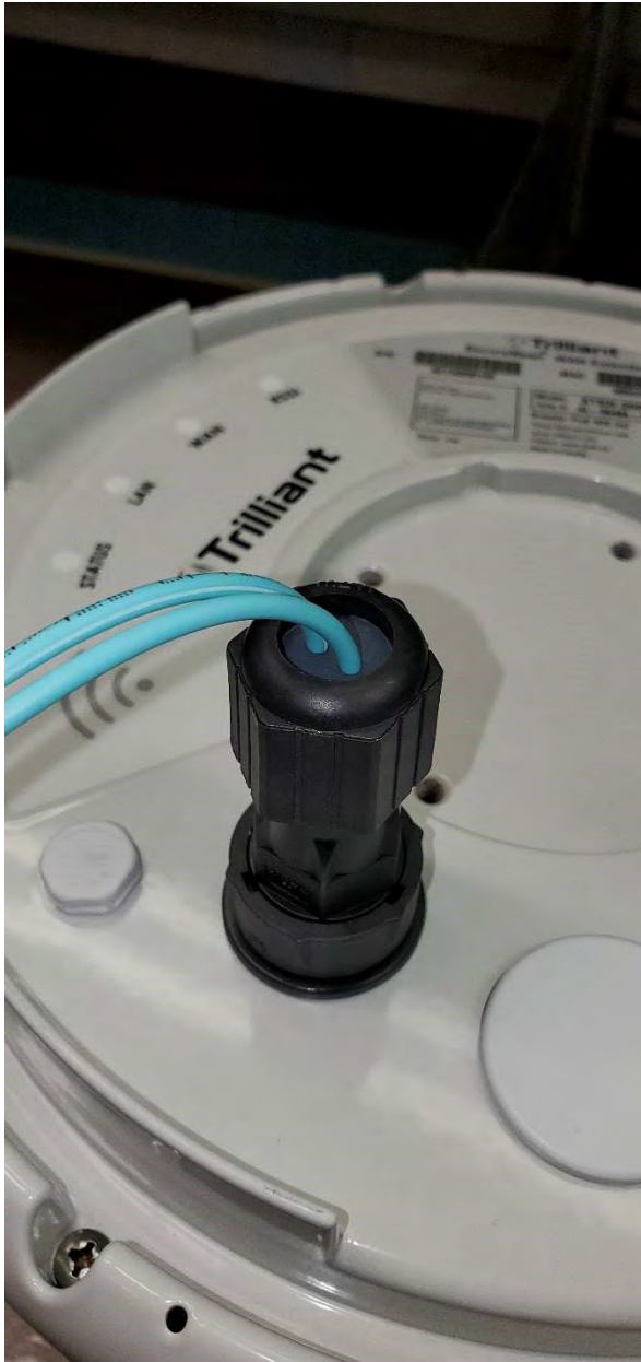
Figure 30: Fiber Optic cable connected to unit with sealing nut.
