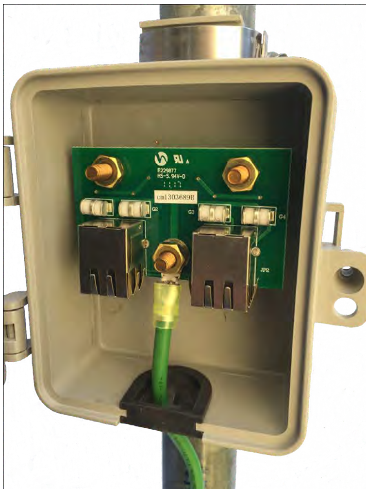
Figure 15: Ground wire installed on surge suppressor
