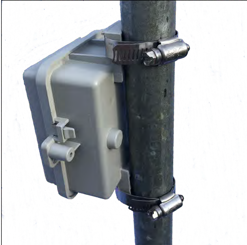
Figure 13: The Citel surge suppressor mounted to the pole
