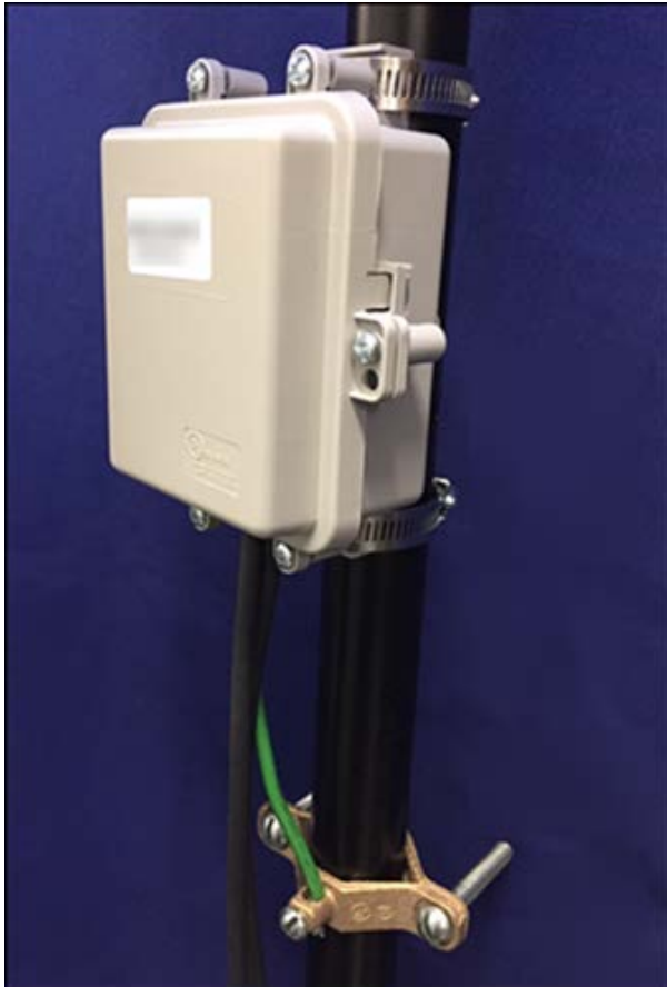
Figure 10: Surge Suppressor Mounted with Ground Clamp
