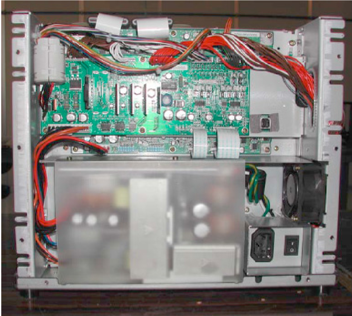
Photograph 13 - Internal Back View of the CV01-H01
