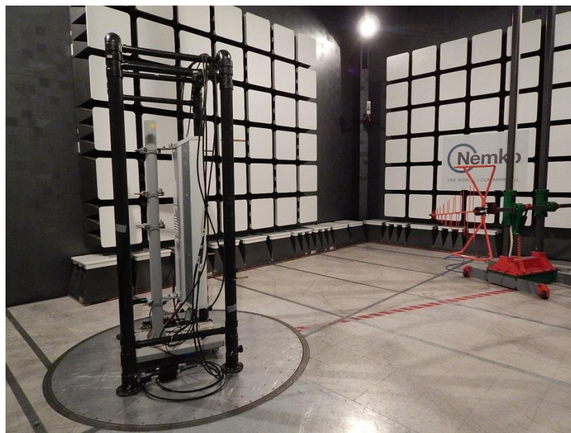
Figure 8.1-38: Setup photo – 30 to 1000 MHz
