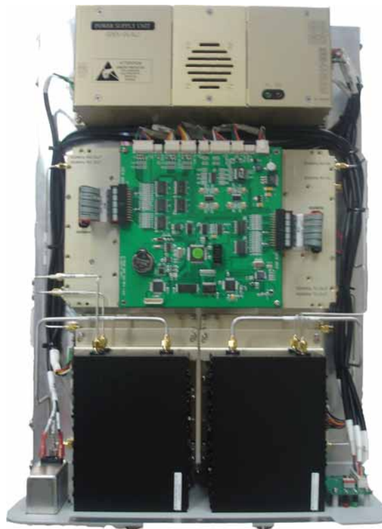
< The Inside of the Repeater >
