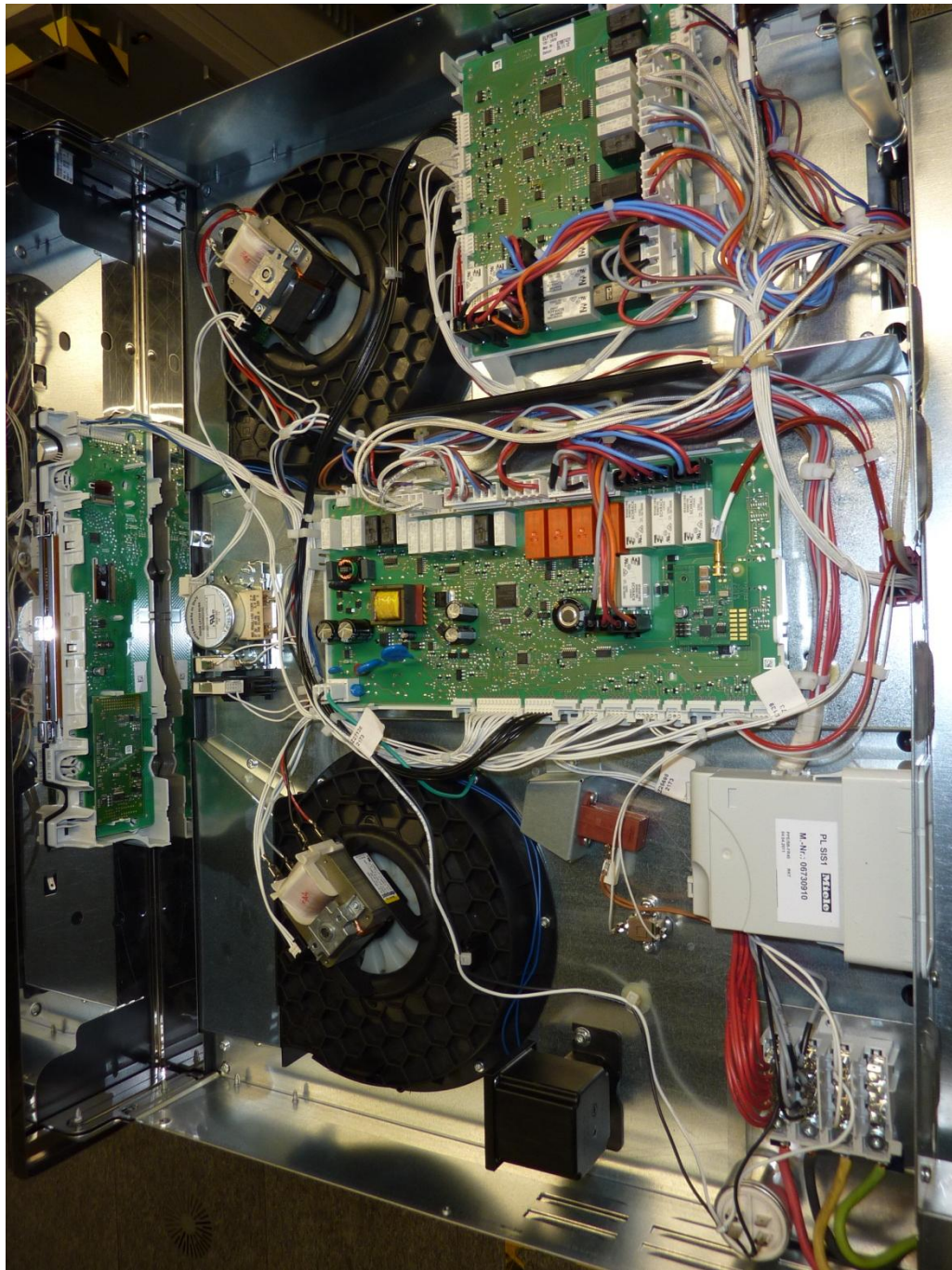
132604_3_e.JPG: EPI7674 inside H6780BP2, internal view 1 (cover removed)
