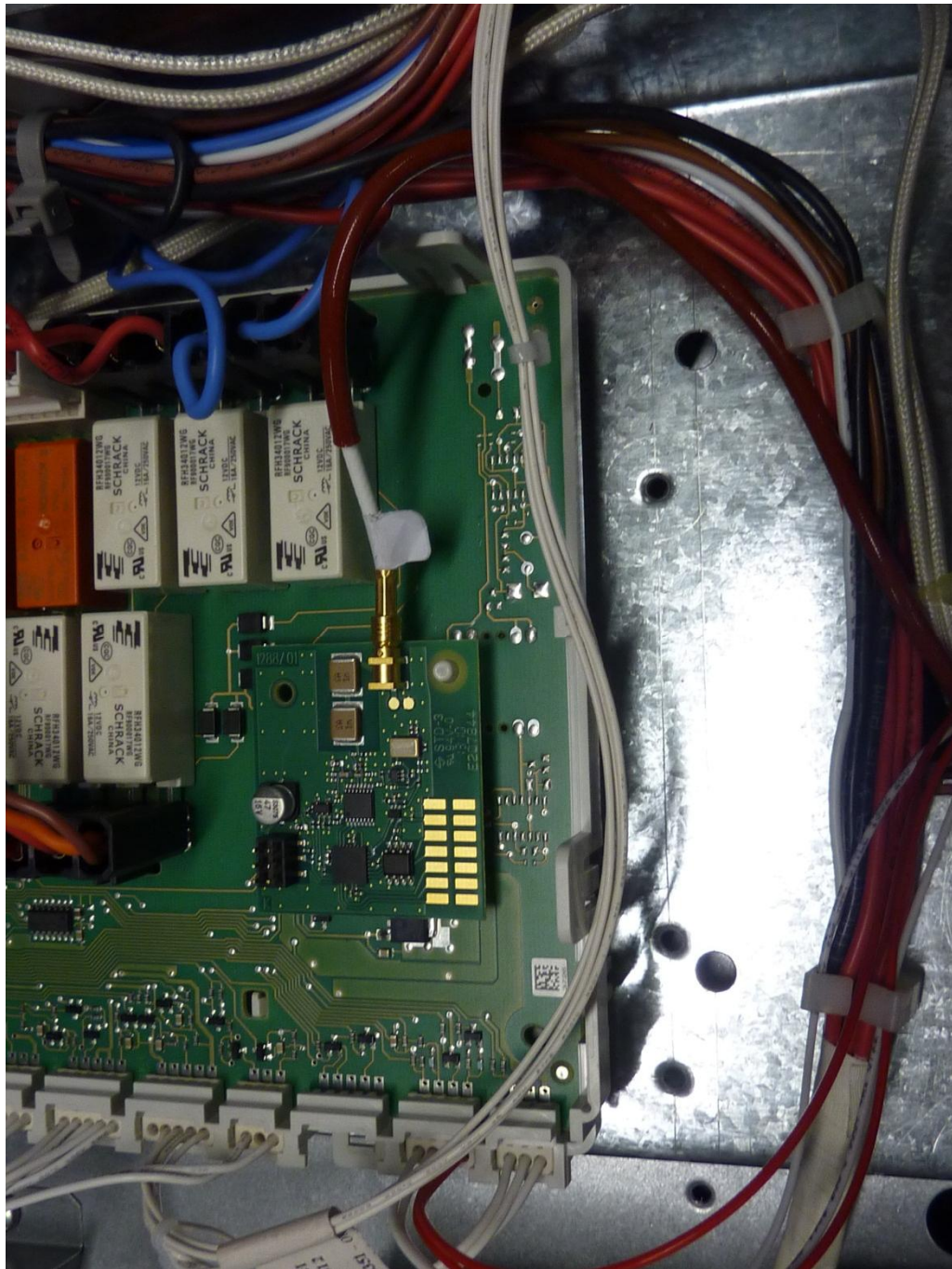
132604_1_m.JPG: EPI7674 inside H6780BP, internal view to rf PCB on main PCB
