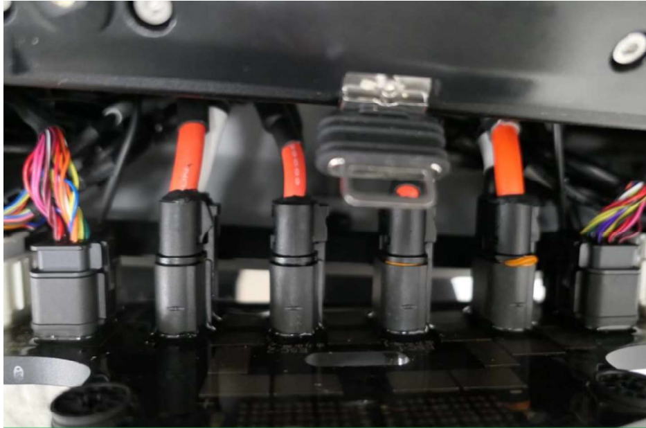
Fig. 31: Internal view for power converter board (for both models)
