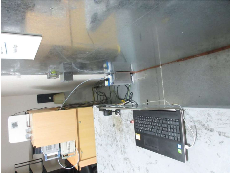
Photograph 9: Set-up for AC Mains (Back View)
