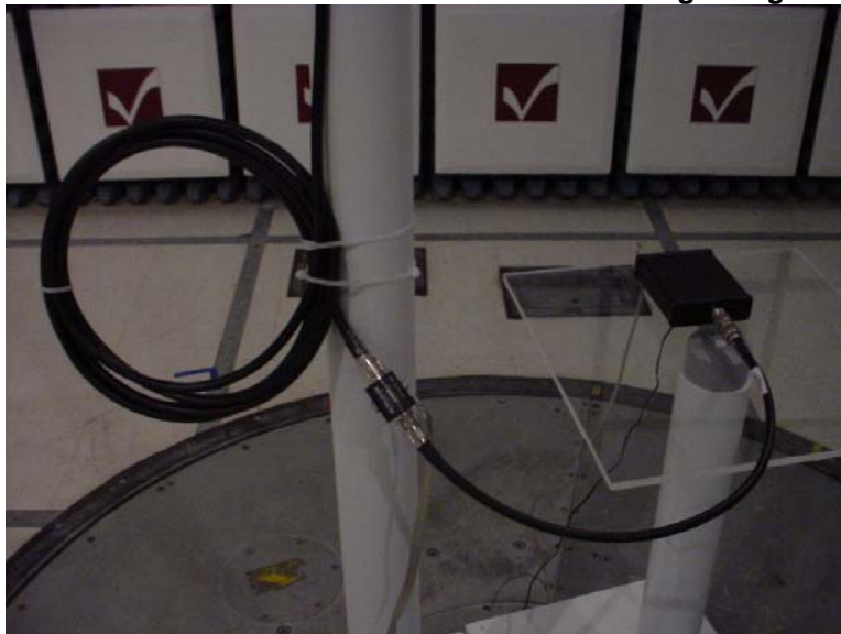
Close-up view of extra cable bundle and the surge protector installation. Surge protector used was an Altelicon model AL-NMNFB Lightning Surge Arrester.
