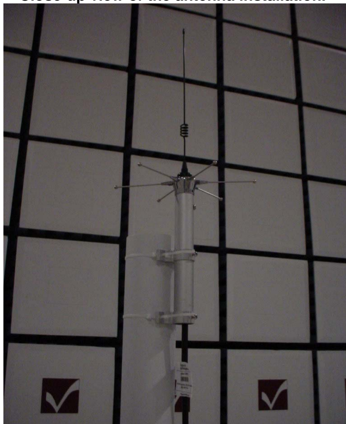
Close-up view of the antenna installation.
