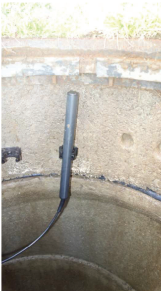
Positioning of a Sigfox antenna
