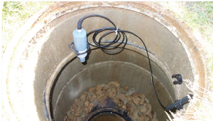
Positioning of a Sigfox antenna 1
