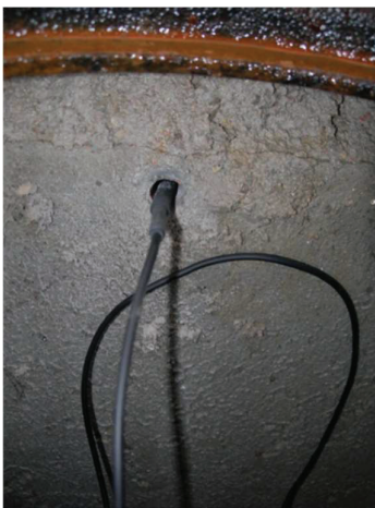
Insertion of cellular antenna in the concrete when sensor install under a manhole cover
