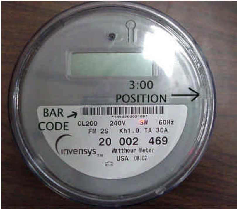
Photograph showing bar code position and 3:00 position for programming wand placement on meter.
