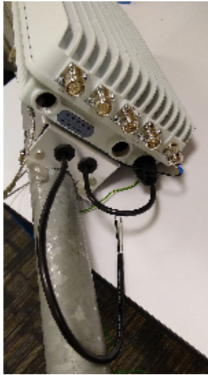
FIGURE 4 Connecting DC Power to the AP
