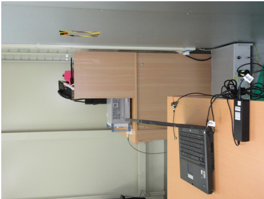
Photograph 10: Set-up for AC Mains (Back View)
