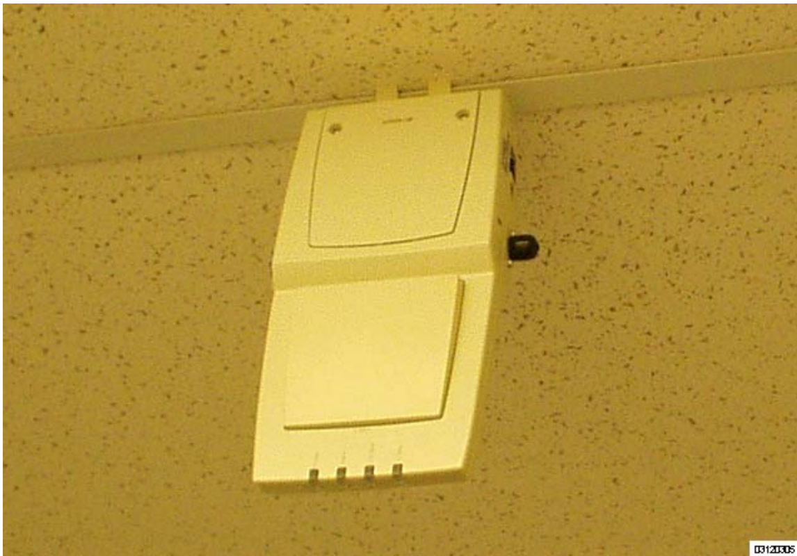
Figure - Clipping the Nortel Networks WLAN - Access Point and Ceiling-Mount Clips to a Hanging-Ceiling Rail
