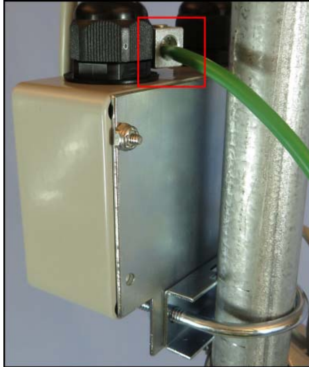
Figure 18 Ground wire on serial surge protector
