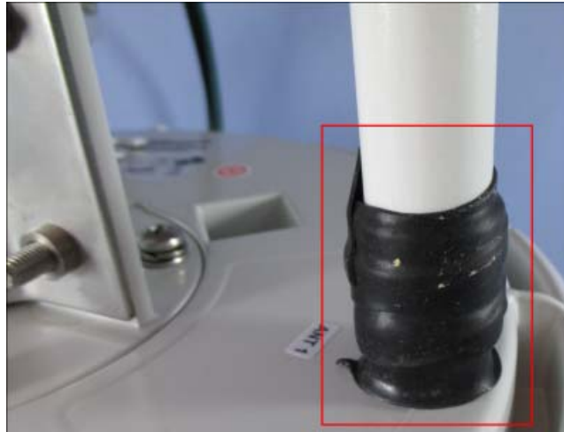
Figure 28 Layer of rubber insulation on antenna connection
