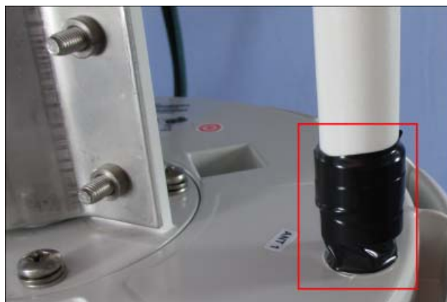
Figure 27 Inner layer of electrical tape on antenna connection
