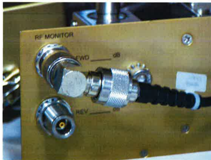
Figure 4-3 RF Monitor Connectors on Junction Box Panel
