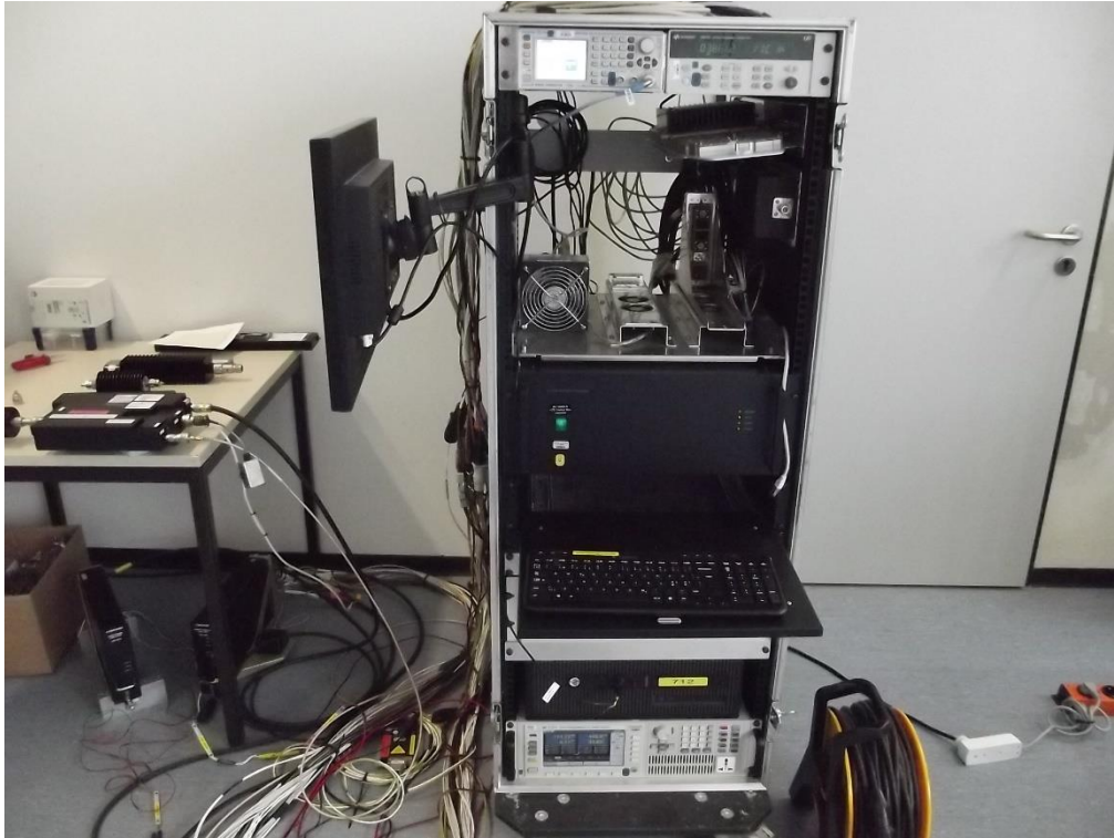
Photo 5: ATS test rack
