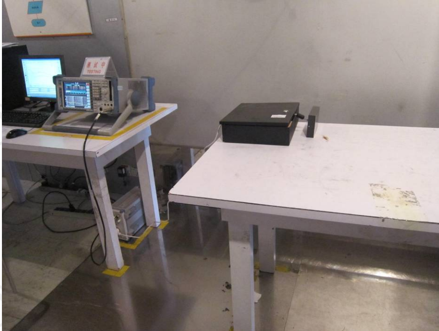
TEST SETUP OF CONDUCTED EMISSION
