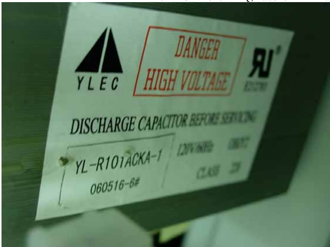
Photo 32 M/N: TSK-M3204MEQ, Label of H.V. Transformer
