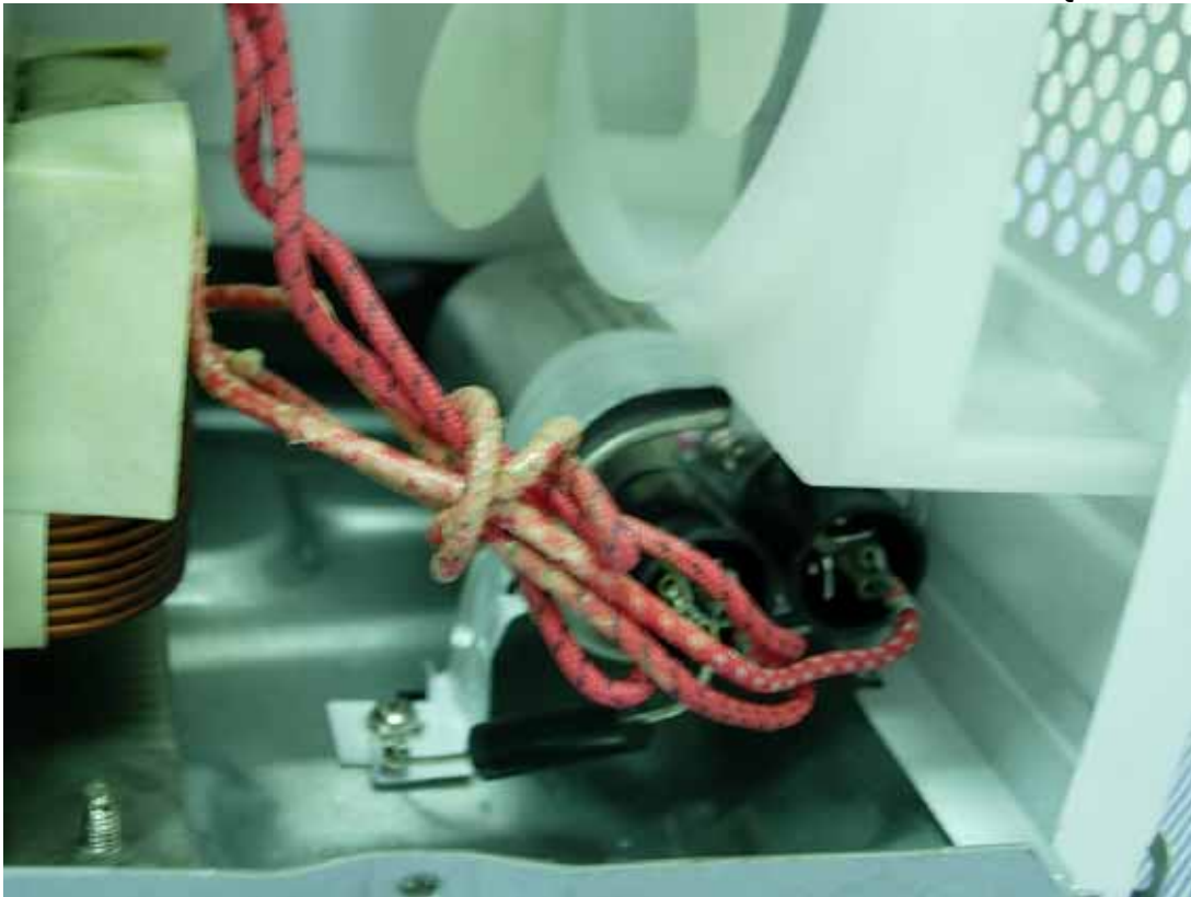
Photo 33 M/N: TSK-M3204MEQ, H.V. Capacitor
