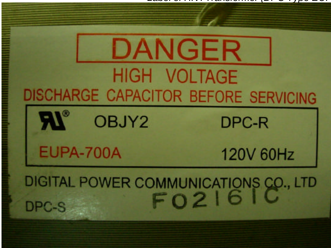
Photo 46 Label of H.V. Transformer (DPC Type EUPA-700A)
