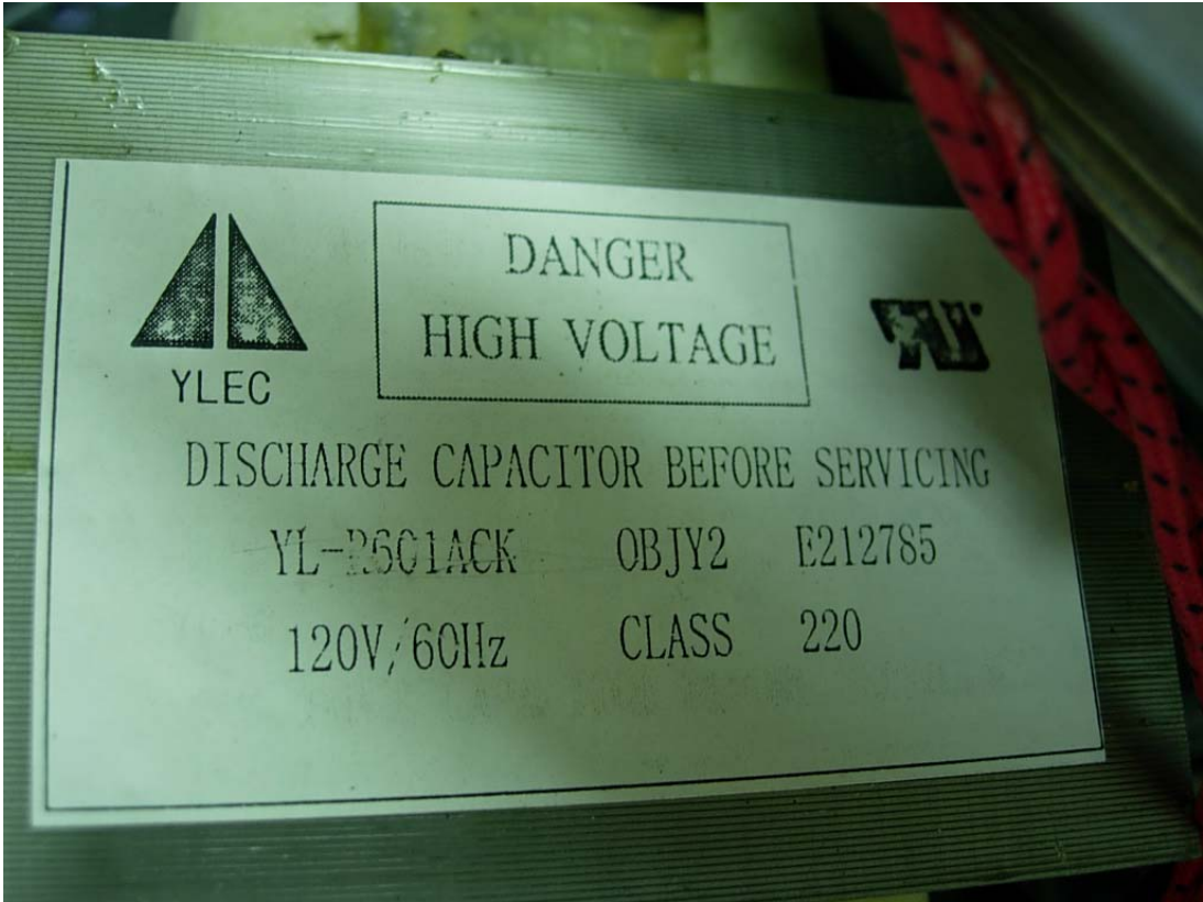
Photo 10 Label of H.V. Transformer
