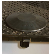
Figure 2.26 Antenna hole in pit lid
