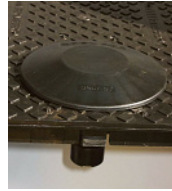
Figure 2.3 Antenna hole in pit lid
