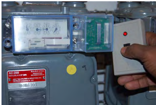
Figure 6 - 23. RF Buster oriented to Gas LX Meter Module for testing
