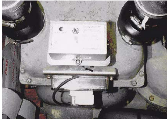
Figure 6.25 Sprague/Actaris: meter with module installed
