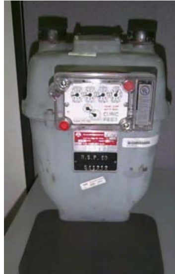
Figure 5.24 Rockwell/Equimeter/Sensus: Correctly installed Meter Module
