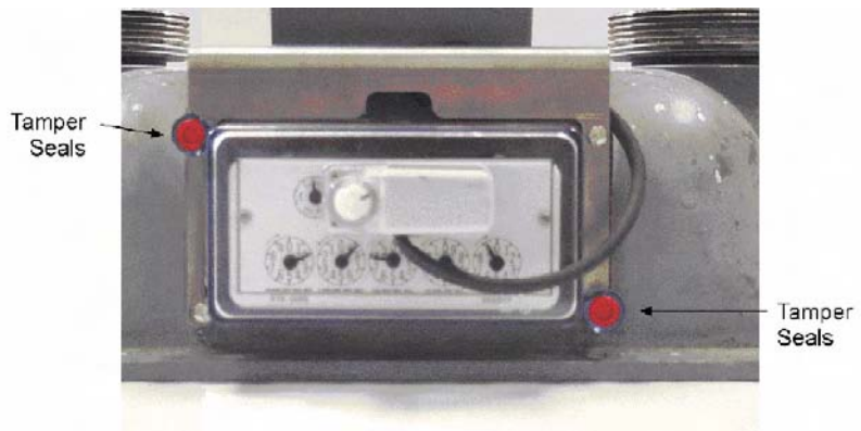
Figure 6.24 Sprague/Actaris: installed tamper seals
