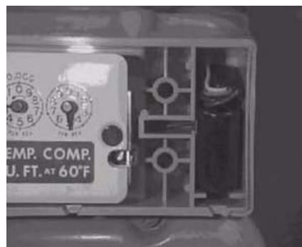
Figure 5.11 American: Properly installed battery
