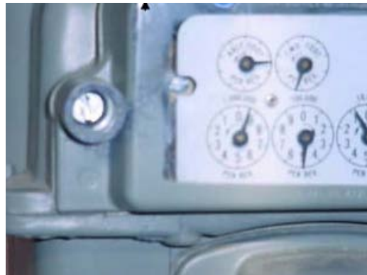
Figure 5.39 Lancaster/National: Meter non-retrofittable
