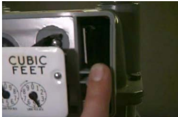
Figure 5.51 Lancaster/National: Battery Correctly Installed
