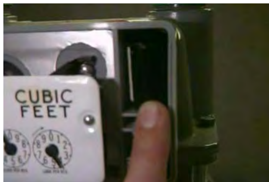
Figure 5.36 Sprague/Schlumberger/Actaris: Battery Correctly Installed
