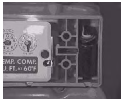
Figure 5.11 American: Properly installed battery
