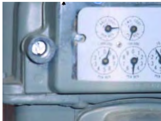
Figure 5.39 Lancaster/National: Meter non-retrofittable
