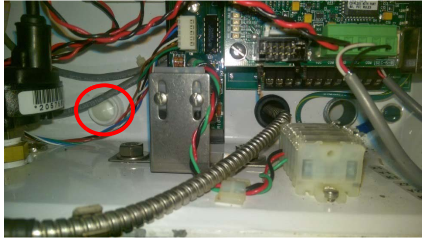
Figure 2 - 9. Mercury ECAT Interior
