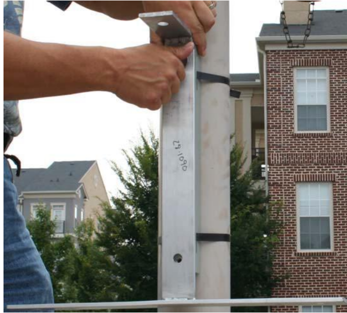
Figure 4 - 5. Antenna light pole bracket attached to mounting bracket
