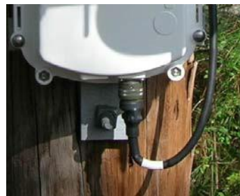
Figure 4 - 1. Cable with drip loop
