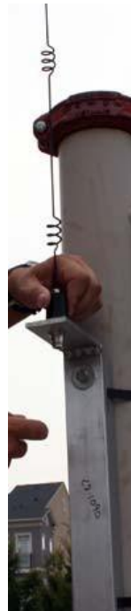
Figure 4 - 7. Connecting the WAN antenna
