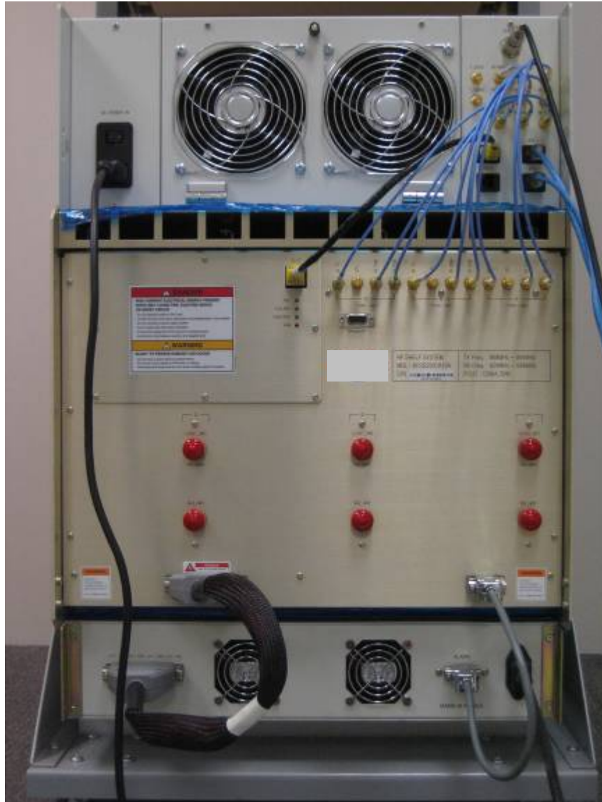
Figure 7-6 Sector RU Field Installation Photograph
