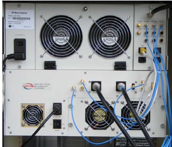
Figure 6-6 – Integrated RU Field Installation Photograph
