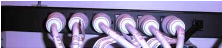
Figure 20 - Electrical Connections in the Powered Auxiliary Cabinet
