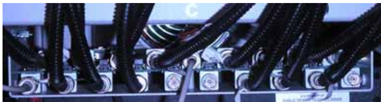
Figure 14 - Antenna Cable to Multiplexer Connection
