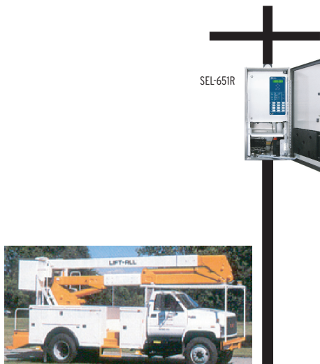
Figure 3.1 Remotely Located Recloser Control
