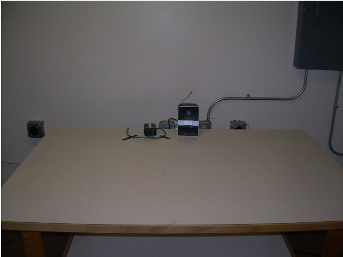
Photograph 8 – Front View Conducted Disturbance Worst Case Configuration – POE Power
