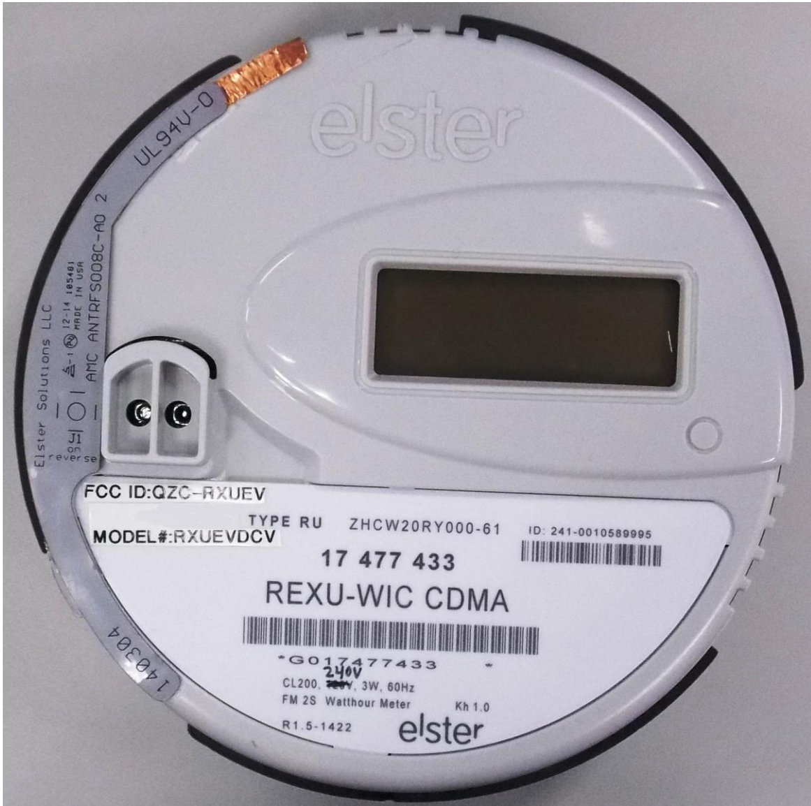
REXUniversal® WWIC cellular antenna installed
