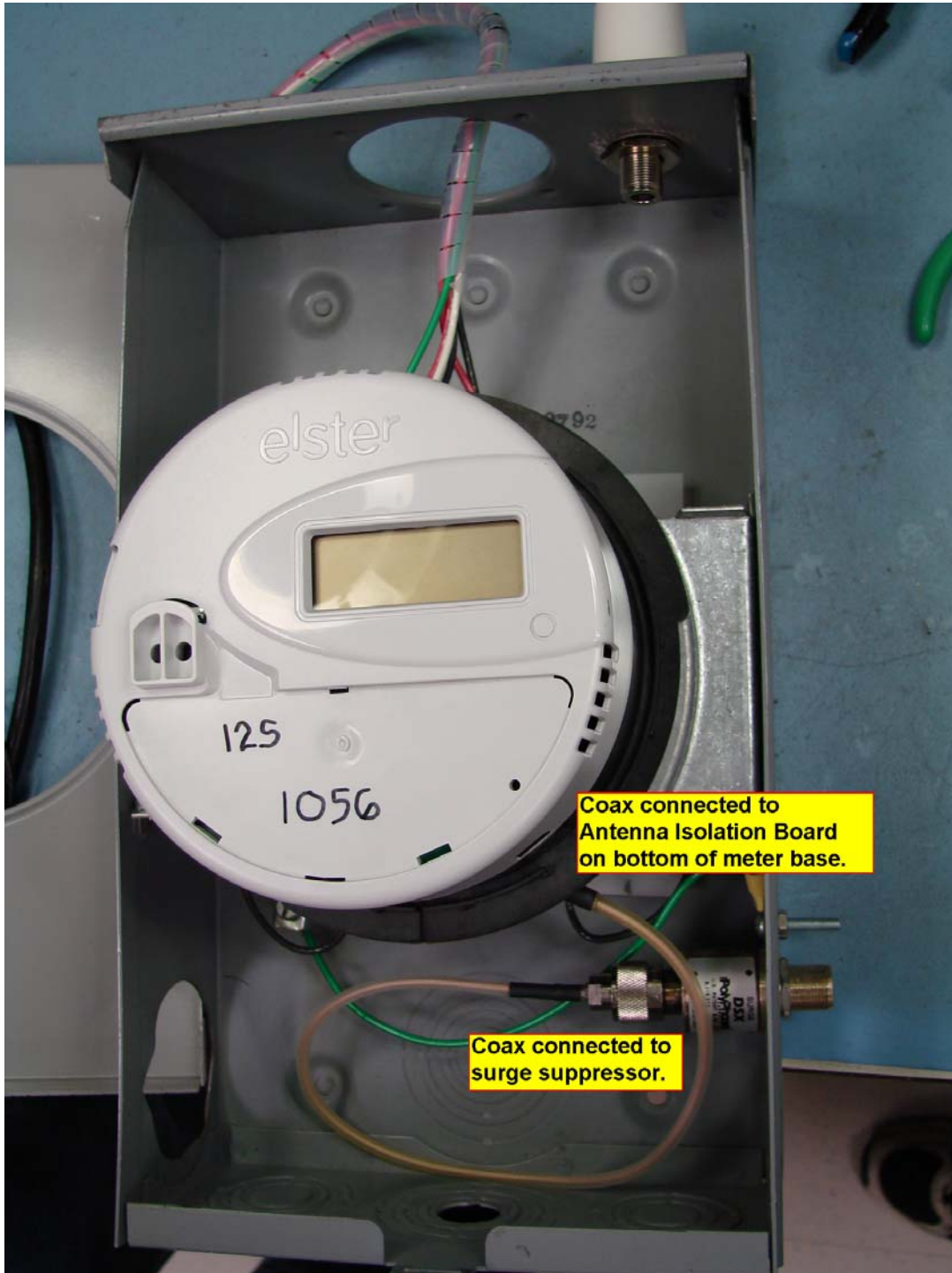
Figure 1: Internal View w/ Remote External Antenna Connection
