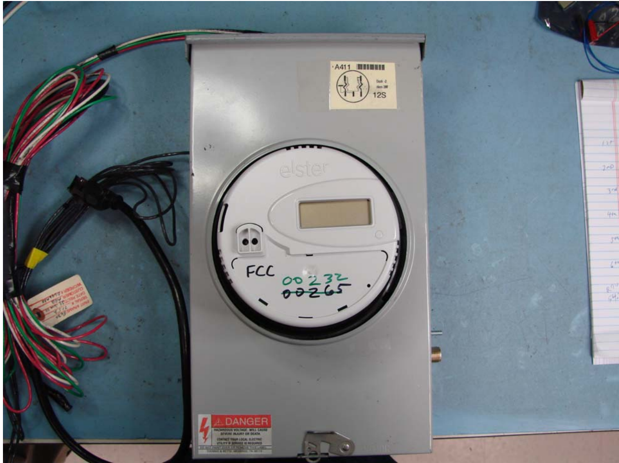
Figure 1: Photo of 12S meter in a 12S electrical socket
