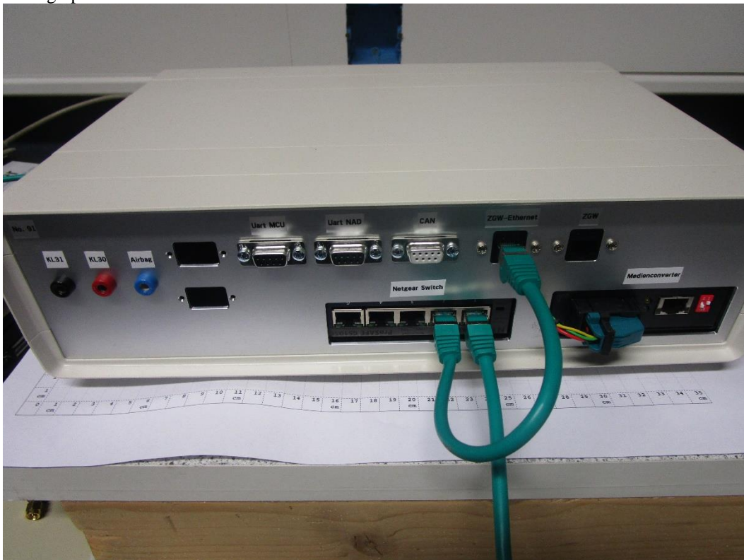
Photograph 12 Connectionbox inside chamber connected with laptop
