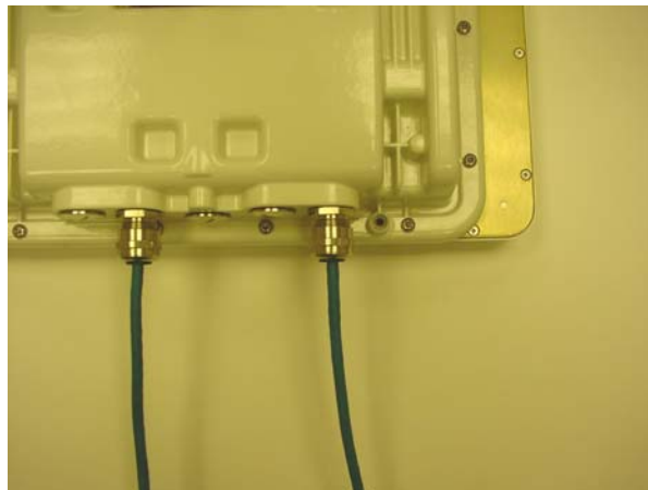
Figure 11 - Making the Network Connection
