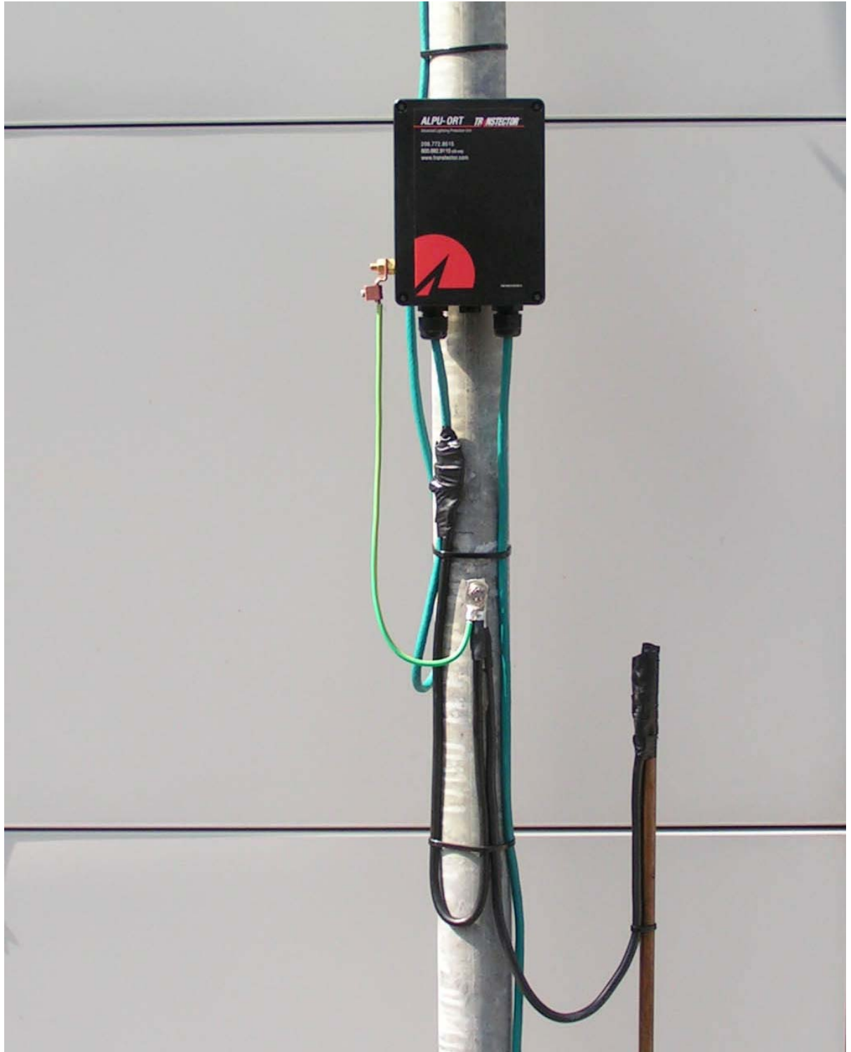
Figure 97 - Lower Grounding Configuration
