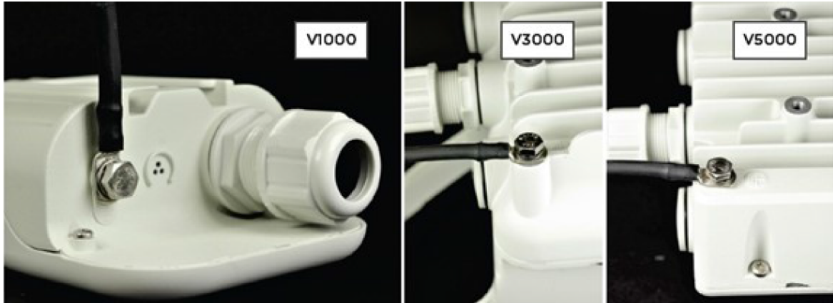
Figure 71: Radio grounding point
