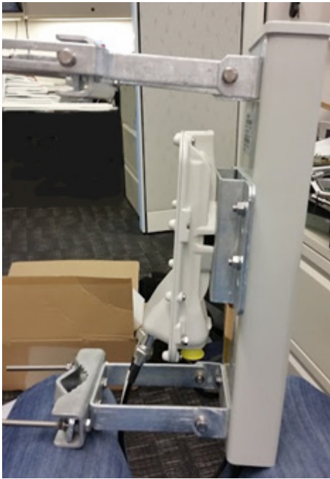
Figure 91 Completed AP and antenna assembly
