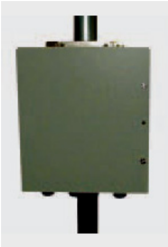
Figure 40 Pole mounted CMM3
