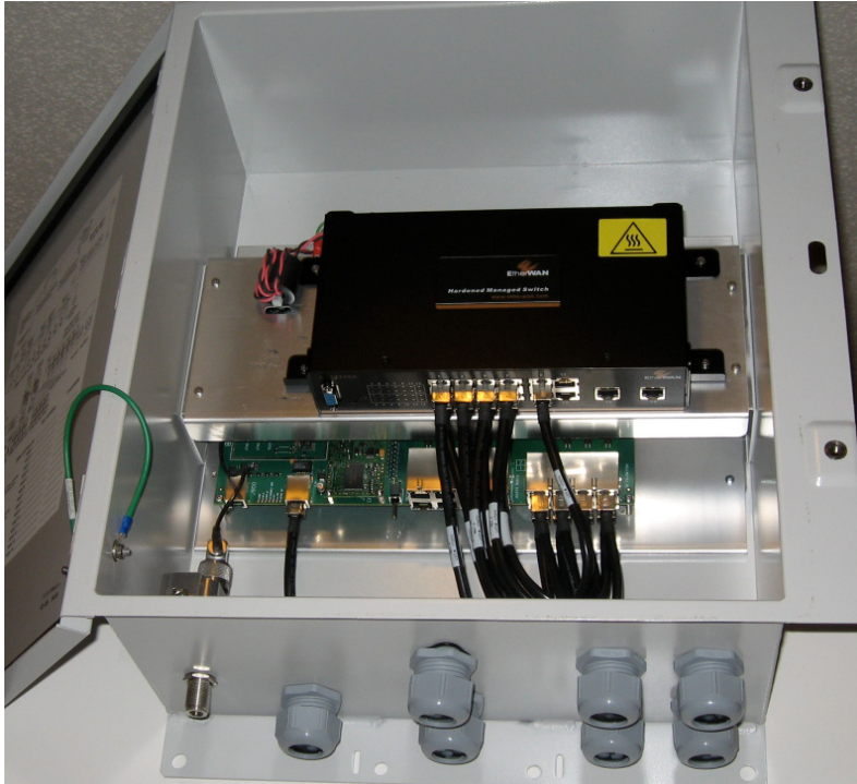
Figure 38 CMM4 (Cabinet with switch)
