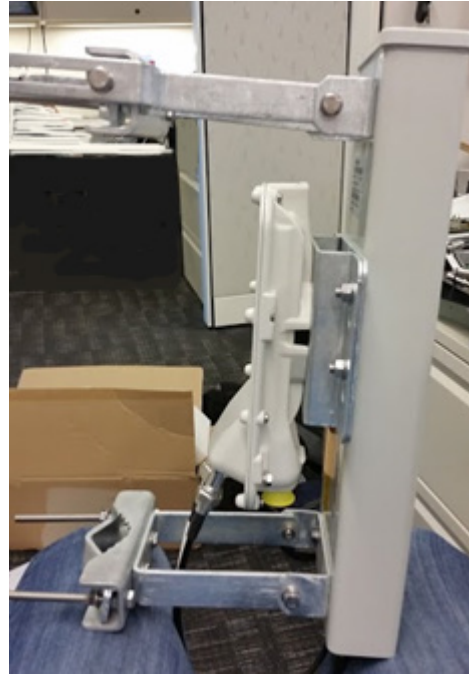
Figure 63 Completed AP and antenna assembly
