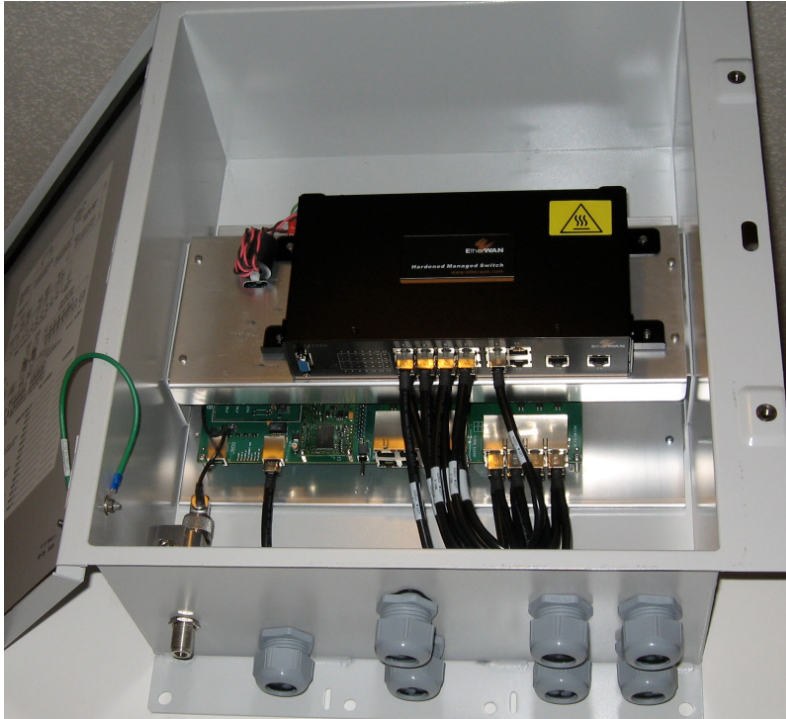
Figure 23 CMM4 (Cabinet with switch)
