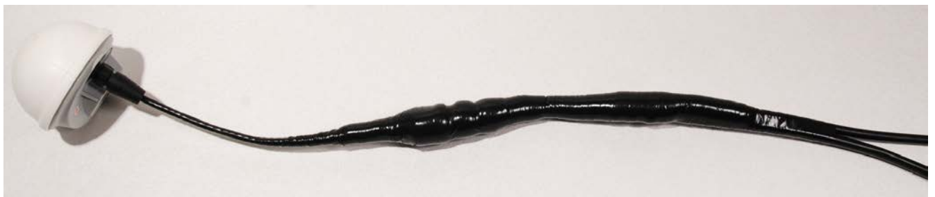
Figure 115 Grounding and weatherproofing example for GPS adapter cable
